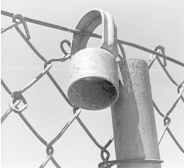
Figure 17 Mounting pole brackets for barbed wire, concertina or razor ribbon not properly secured to the fence posts
