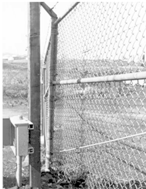
Figure 14 Loose fabric at diagonal stiffeners
