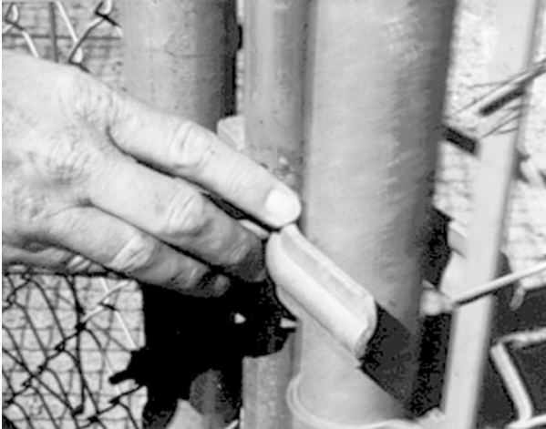
Figure 19 Excessive play between locking posts and metal insert
