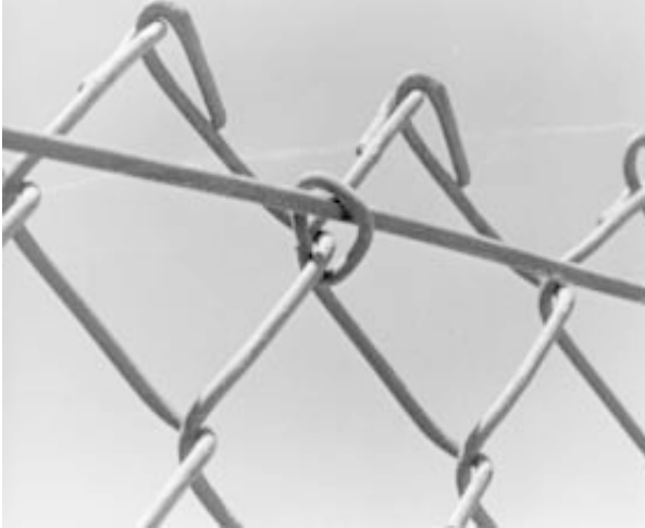
Figure 15 Loose fabric or clamp rings at steel wire stiffeners
