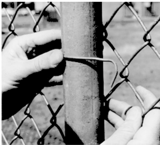
Figure 13 Loose fabric at fence posts or horizontal rails
