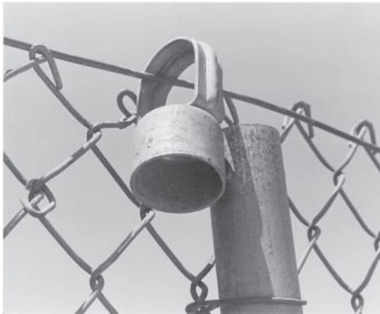
Figure 16 Mounting pole brackets for barbed wire, concertina or razor ribbon not properly secured to the fence posts
