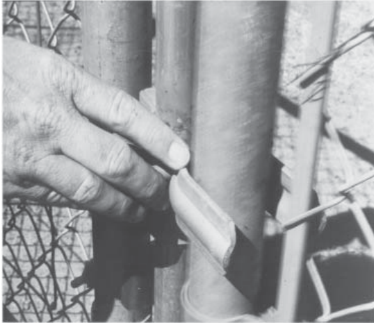
Figure 18 Excessive play between locking posts and metal insert
