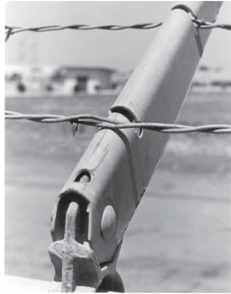
Figure 15 Barbed wire dangling due to missing keepers
