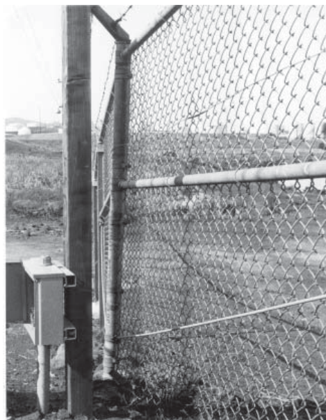
Figure 13 Loose fabric at diagonal stiffeners
