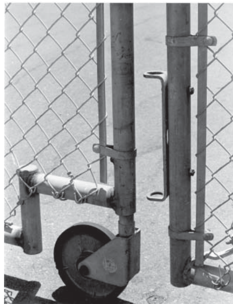
Figure 17 Missing vertical locking posts
